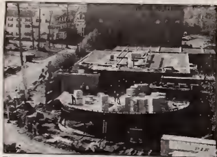
The Mater Building construction is slated for completion late next summer. The building will be the new home for the School of Hotel, Restaurant, and Recreation Management, and will include the school's dining room, production and research kitchens, classrooms, technology center, audio, hospitality information systems lab, and offices.
